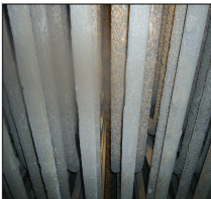
Fig. 7. Clogging phenomenon on outer wall of water pipe: (a) case of leachate, (b) case of food wastewater
