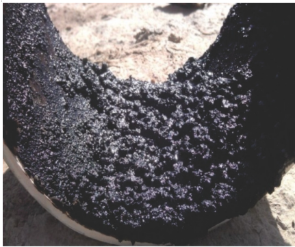
Fig. 1. Sediments in pipeline
