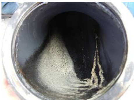
Fig. 4. Urea crystallization and sedimentation phenomenon on the inner wall of the exhaust pipe
