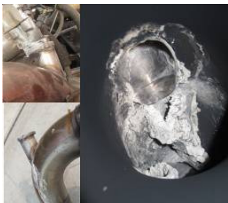
(a) Bottom of the injector mounting base
